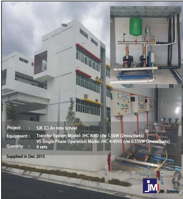
Year 2015 – Transfer System & Single Operation (6 sets) At SJK (C) Jln Imbi School
