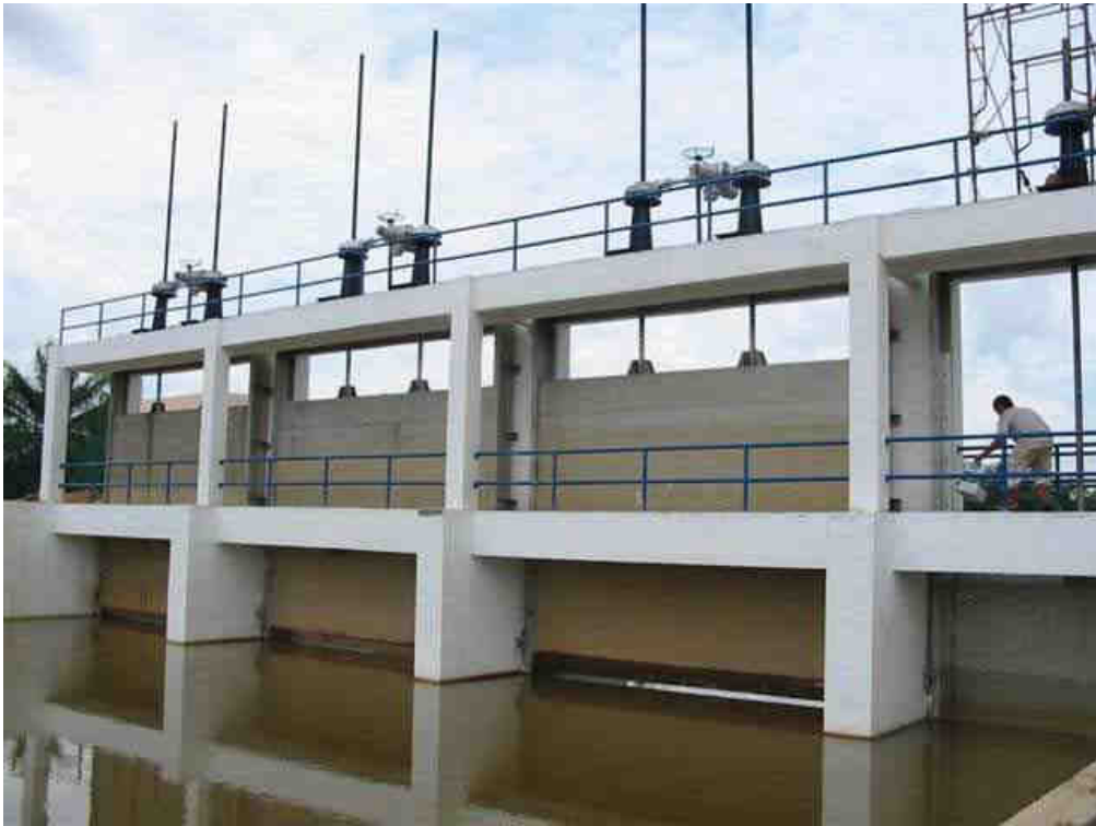
Sungai Bogak Pump House Gate (5m x 4m)
