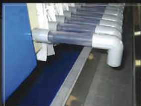
Filtrate Diversion Tank.
