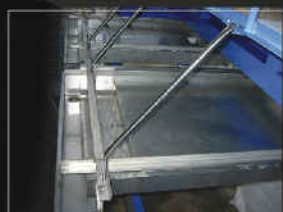
Stainless Steel Water Gate.
