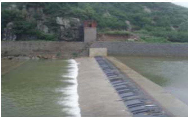
Deflation of Crest Gate with Rubber Dam
